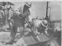
BEFORE DOWELS cover the openings, the area must be drilled to size, far left, and the bolt fixed, left. The twelve-by-twelve-inch timbers are picked up and positioned by a crane after the bolt and dowel holes have been drilled. Holes are visible in the timber above.
